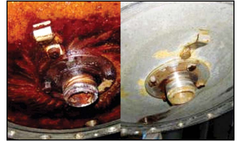
Vessel cover contaminated
